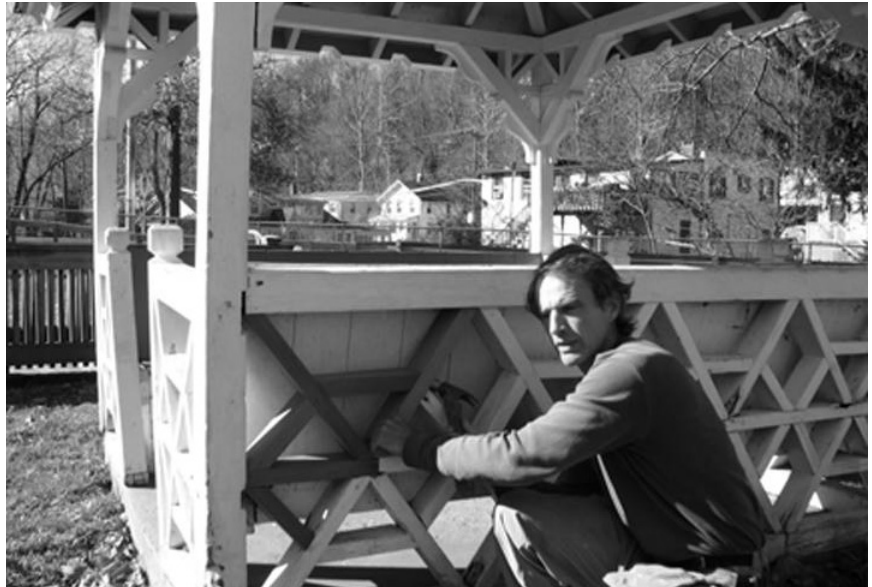
Carpenter Michael Brennan repairs the Kane Park gazebo. The Piermont Civic Association built the gazebo many years ago and has maintained it ever since.
